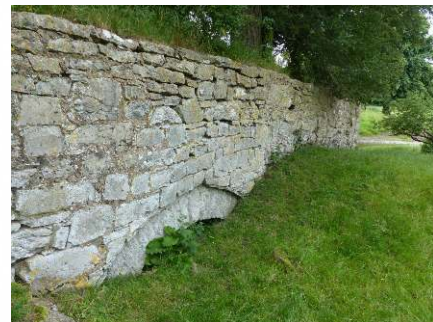
This arch of Tunnel Bridge spanned the old mill leat and is thought to be medieval.
